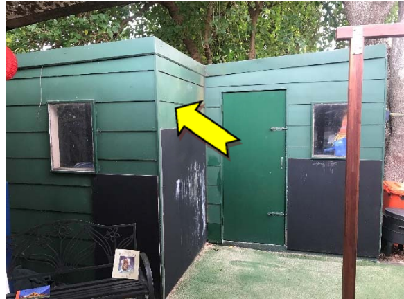
Photo 2. Exterior, throughout, wall paneling – suspected lead-containing green upper paint system.
